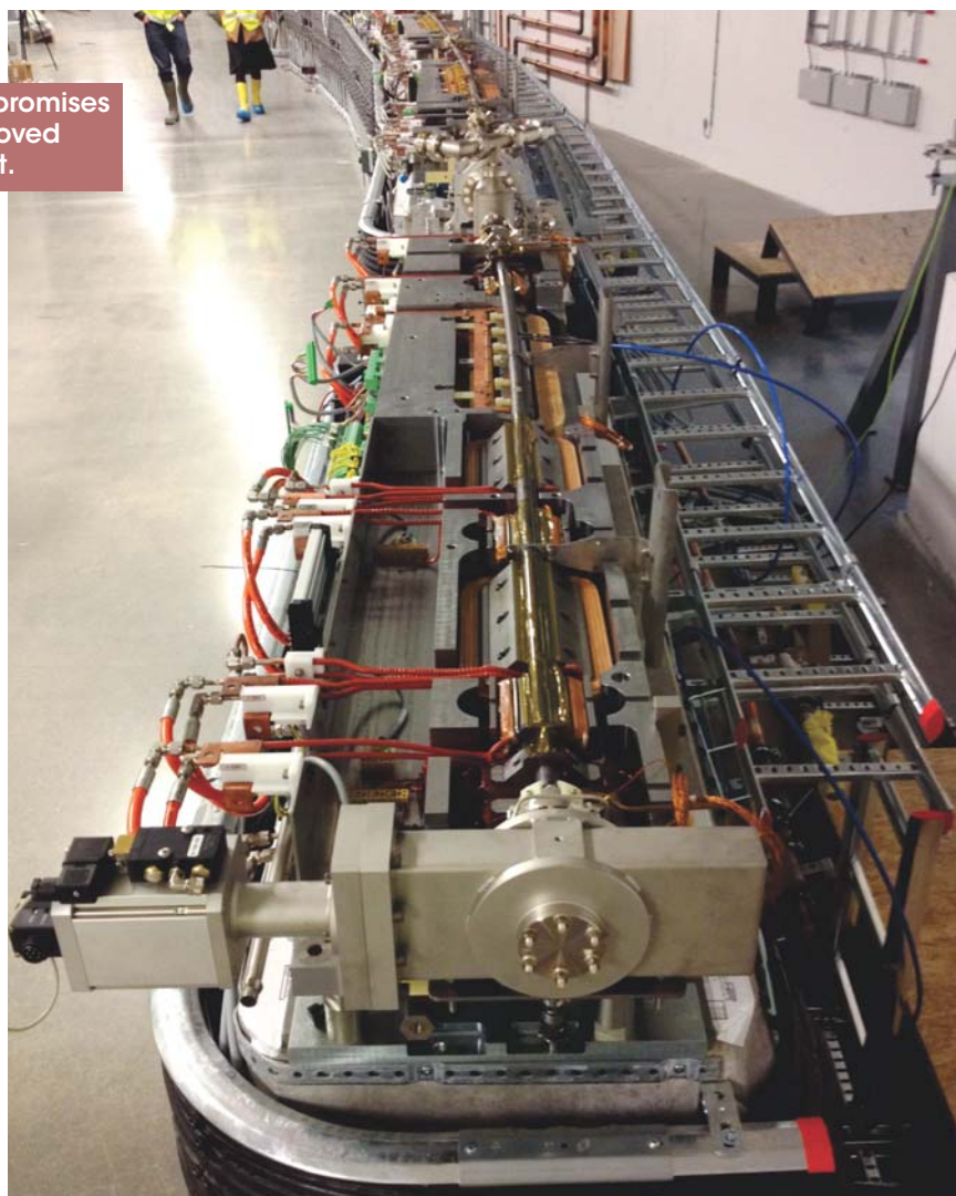
The large storage ring at the MAX IV light source in Lund, Sweden, has 20 seven-bend magnets; the lower half of one is shown here. The upper half will be added as the final installation step. Carving the magnets into iron blocks cuts costs and simplifies the alignment process.
