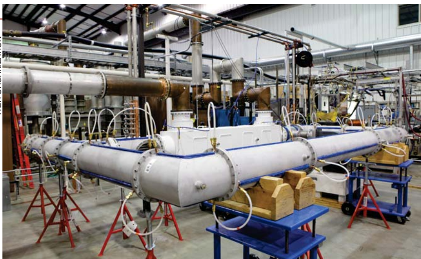
This test stand at Oak Ridge National Laboratory will demonstrate that a US contribution of large-scale 12-inch coaxial transmission lines for ITER's ion cyclotron heating system can perform to specifications.
