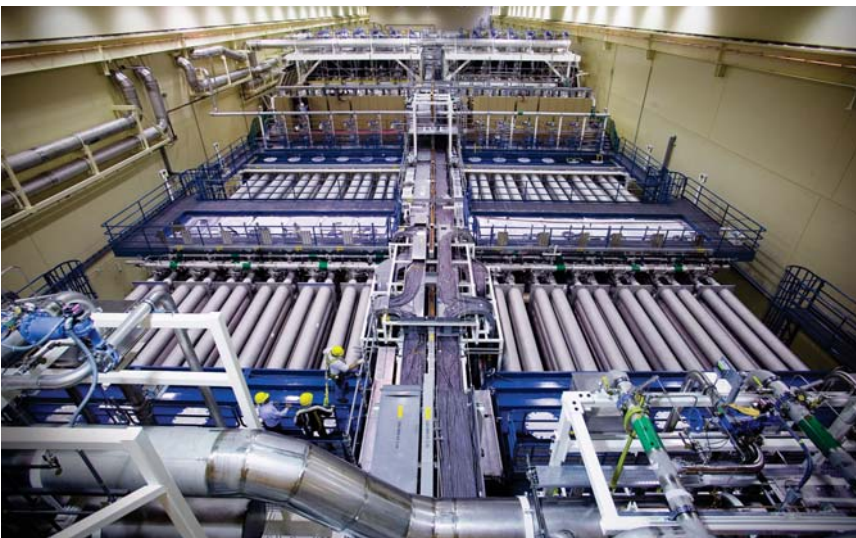
Seen from above , each of the National Ignition Facility's two identical laser bays has two clusters of 48 beamlines, one on either side of the utility spine running down the middle of the bay.
