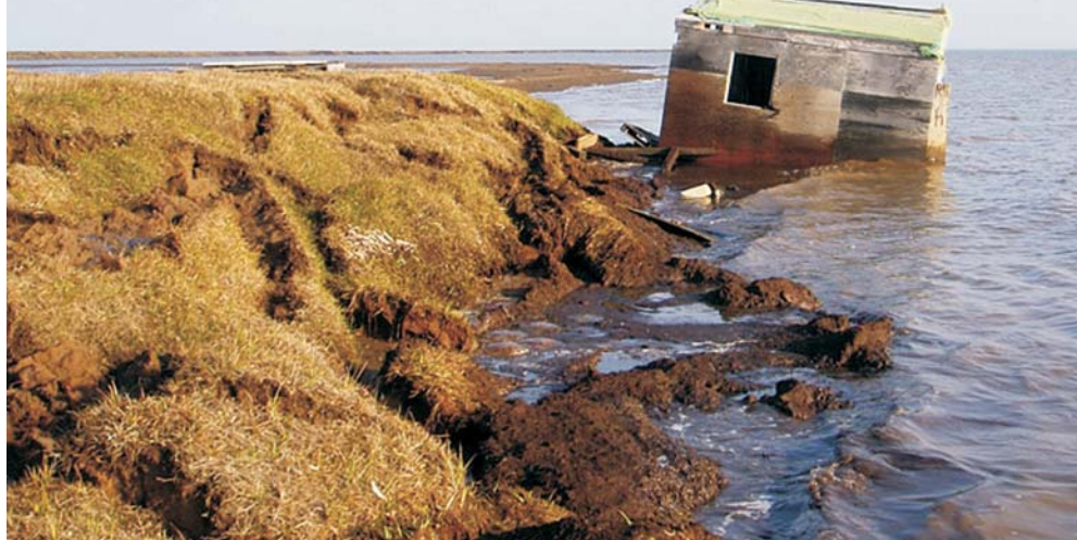
Figure 1. A cabin along the Alaskan coastline has collapsed into the Beaufort Sea because of coastal erosion. Warming sea temperatures, rising sea levels, exposure to choppy waves, and the thawing of ice-rich bluffs have contributed to an increase in the erosion rate—from 8.7 m/year between 1979 and 2002 up to about 14 m/year between 2002 and 2007—along a stretch of that coastline. 5 (Photo courtesy of Benjamin Jones, US Geological Survey.)
