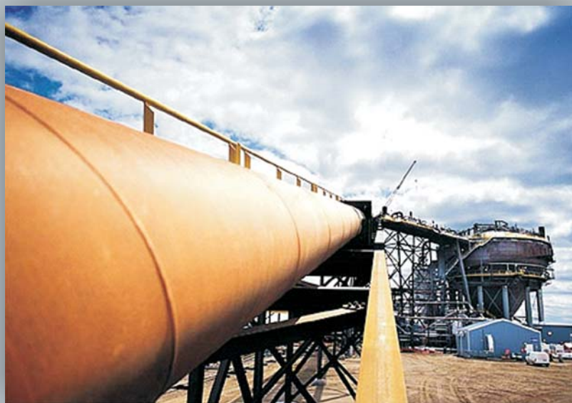
Figure 3. The hydrotransport pipeline
