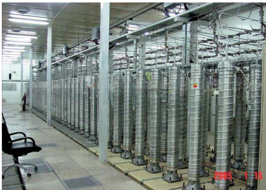
Figure 3. The first publicly released picture of the 164-machine cascade installed at Iran's aboveground Pilot Fuel Enrichment Plant. The photo was used in a presentation by Mohammad Saeidi of the Atomic Energy Organization of Iran in September 2005.
