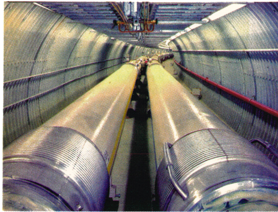
TWO RINGS OF CRYOSTATS house the superconducting magnets that carry RHIC's heavy-ion beams, in opposite directions, on their collision course. The view is one of the arc sections of the RHIC tunnel. (Photo courtesy of Thomas Ludlam, Brookhaven National Laboratory.)
