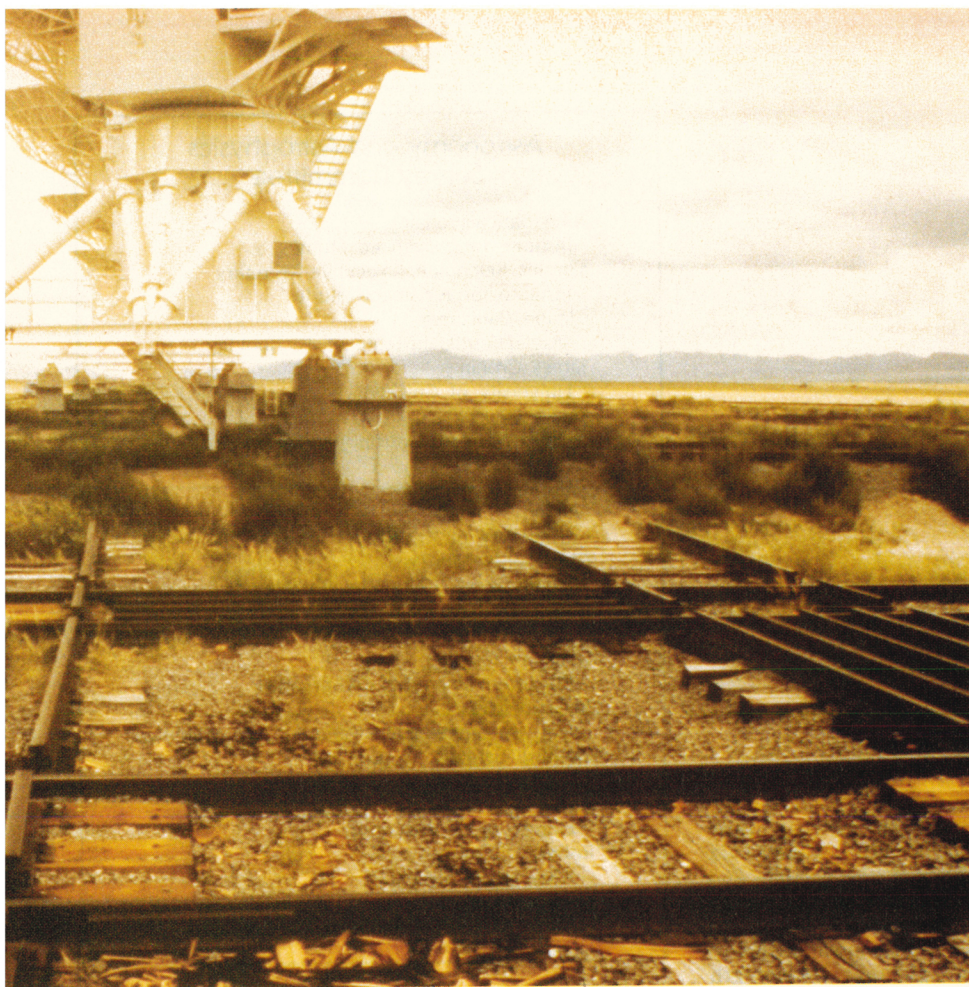
A decade of deferred maintenance and refurbishment has led to a variety of problems at the national observatories, including the deterioration of the railroad track used to reconfigure the Very Large Array for operation at different spatial resolutions. (Courtesy of the National Radio Astronomy Observatory—Associated Universities.)
