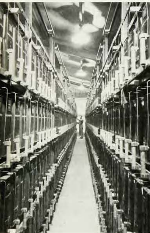
Capacitor bank for Berkeley synchrotron was assembled from surplus units at other installations. Figure 3
