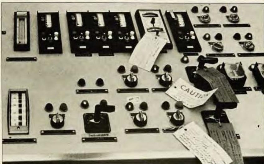
Maintenance tags on TMI-2 control panel covered one of two lights indicating that the two emergency feedwater valves were closed. No one knows why the second light was missed. The closed valves were discovered eight minutes into the accident. Photo courtesy Metropolitan Edison.
