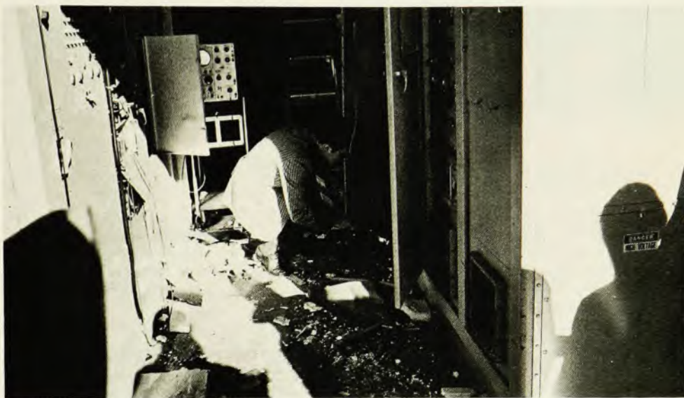
Damage caused by the explosion of two bombs in the klystron gallery of the Stanford Linear Accelerator Center is inspected. The accelerator itself was only slightly affected.
