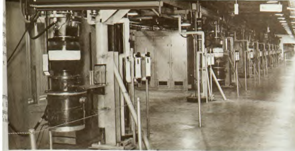
KLYSTRON GALLERY AT SLAC. The two-mile gallery has a 24-MW S-band klystron every 12 meters. On the shelf above and to the right of the first klystron is one of the 120 ion-getter vacuum pumps.
