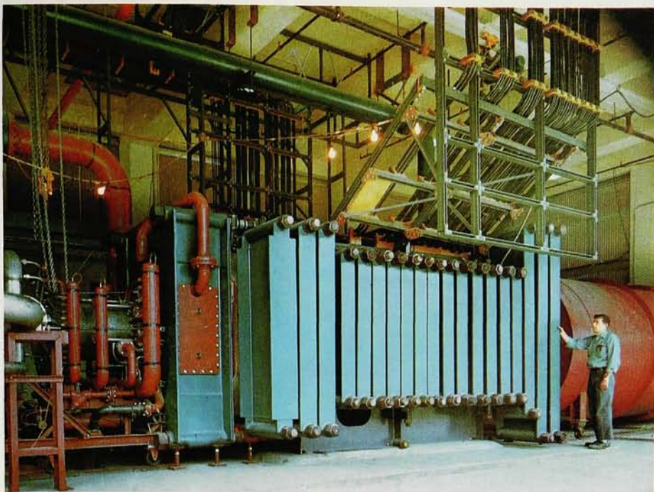
AVCO MARK V MHD GENERATOR produces a dc output of 31.3 megawatts. It is a rocket-driven device with a self-excited magnet, requiring no outside power.
