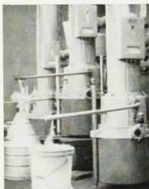
Plant Photograph Nitrogen Cryogenerator units
