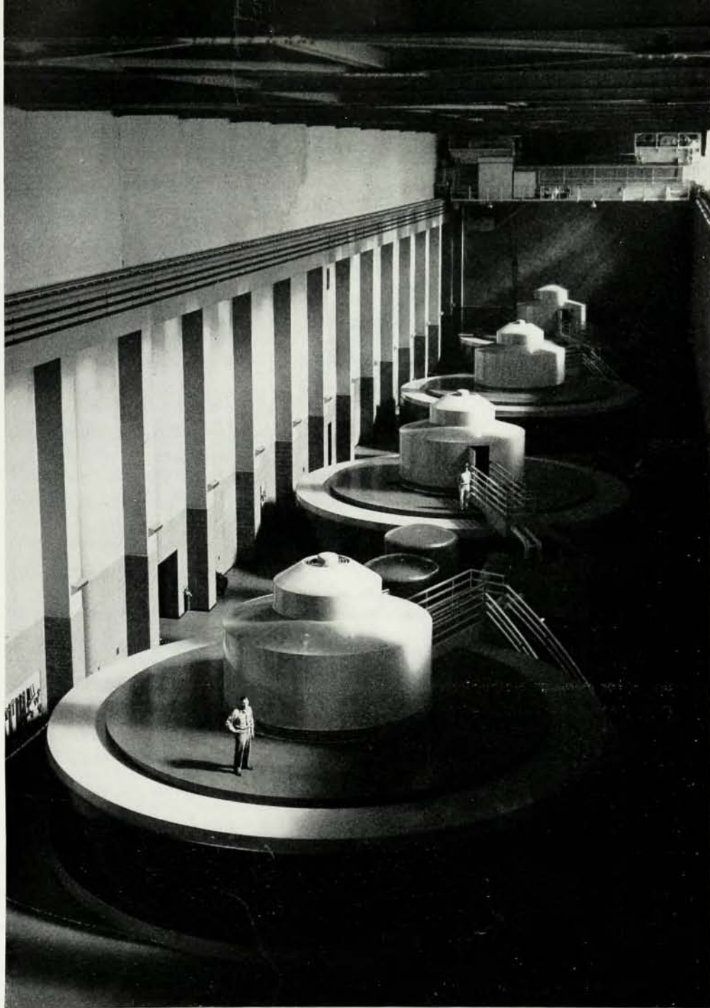
Generators in the power house of Pickwick Landing Dam, T.V.A. Ewing Galloway
