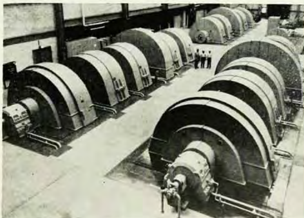
Fig. 5. The three large motor-generator sets (each with flywheel) used to power magnetic field of the C Stellarator.
